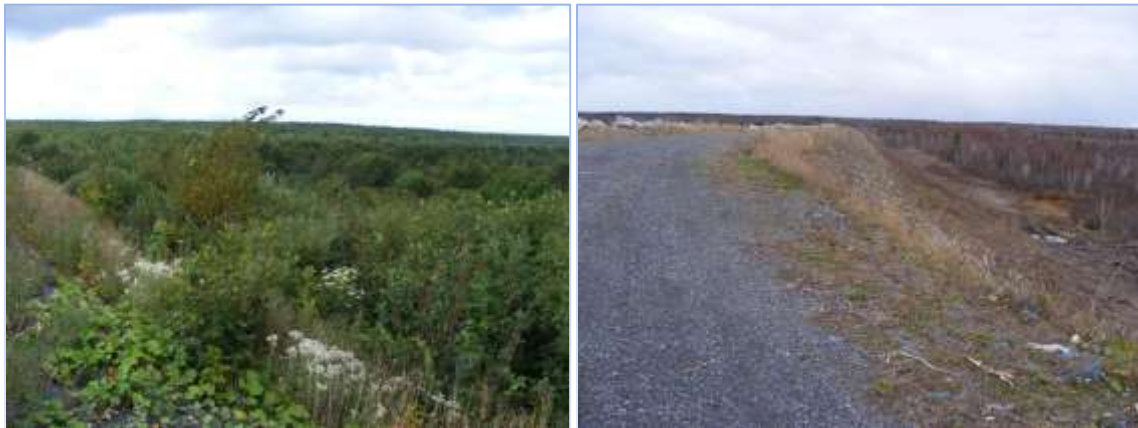
Figure 5. Dam face September 2008 on left and November 2010 on the right
