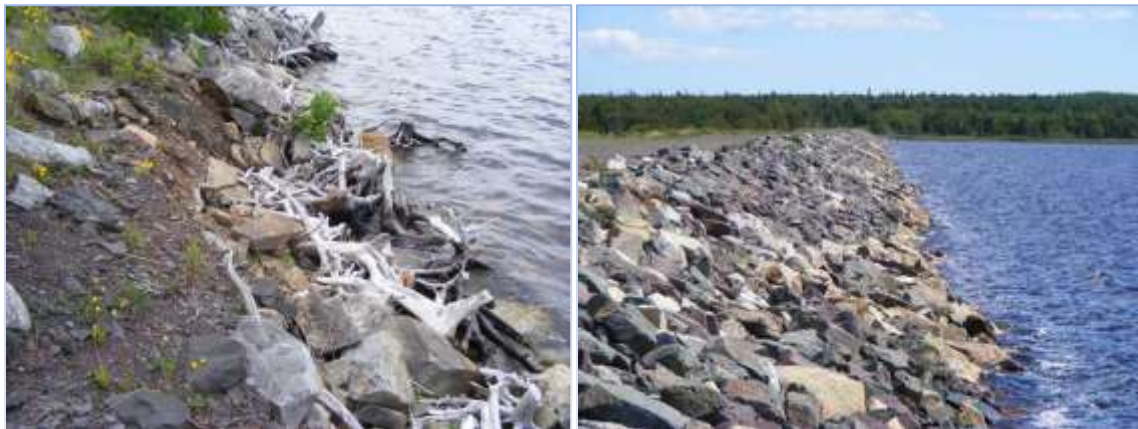
Figure 7. Missing rip rap June 2009 and same section following repair August 2011
