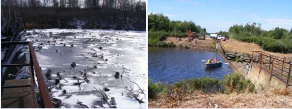
Figure 4. Stumps blocking spillway January 2010 and being removed September 2010
