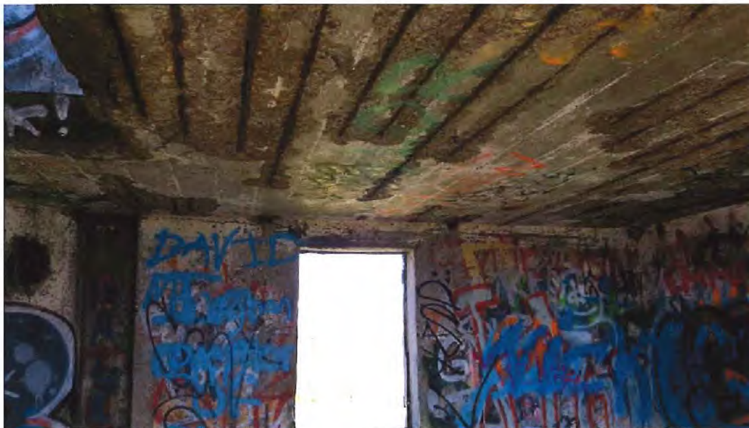
Spalled concrete and exposed rebar which is typical at the underside of floor slabs
