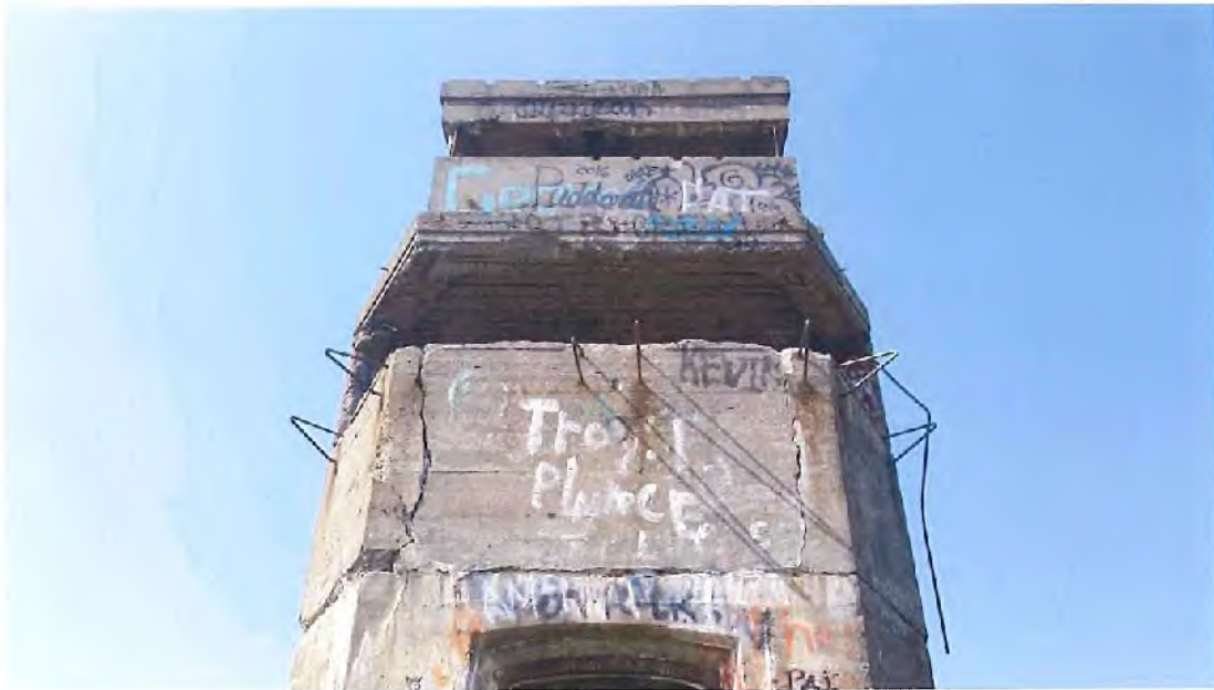
Cracked concrete walls and exposed rebar at underside of floor slabs
