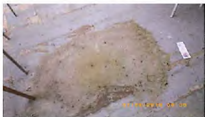
Rat Droppings on floor
