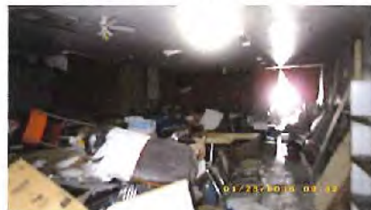
Large amount of combustible material in rear storage room
