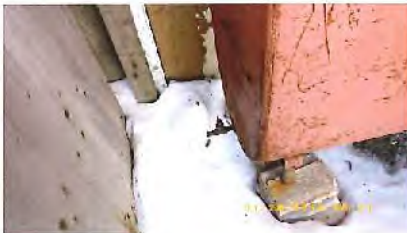
Connection at Oil tank Shut off Valve Broken
