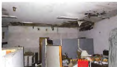
Mold on ceiling
