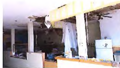
More holes in ceiling
