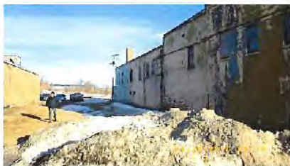
Side of Building depicting Deterioration of Wall
