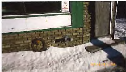
Sprinkler Connection not In Service
