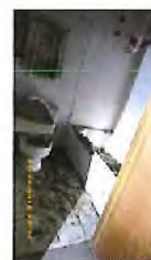
Insulation falling from ceiling into bathtub
