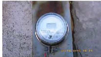
Power Meter showing Power not being supplied
