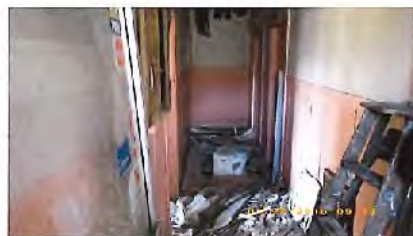
Large holes in upper level floors very dangerous
