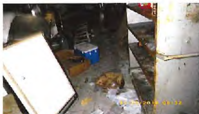
Junk in Storage room
