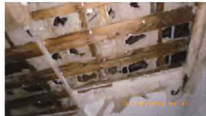
Ceiling missing in storage room
