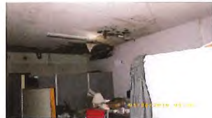
Ceiling full of mold
