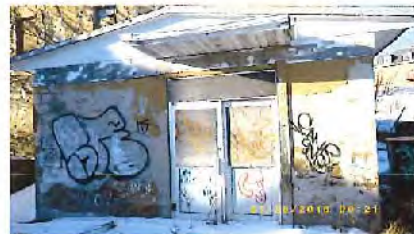
Graffiti At rear of Building
