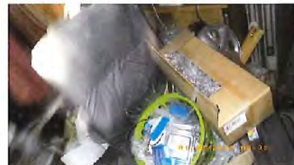
Combustible material in storage room
