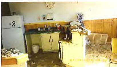
Kitchen area depicts blown in insulation that has fallen from ceiling
