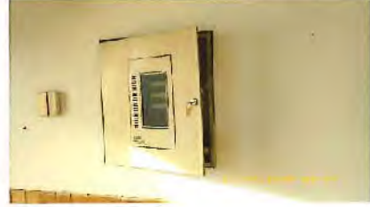
Fire Panel not functional
