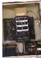
Fire Panel not operational
