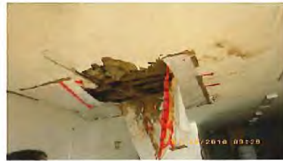
Hole in ceiling
