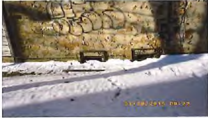
Opening allowing Vermin to enter building
