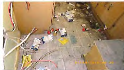
Electrical System vandalized
