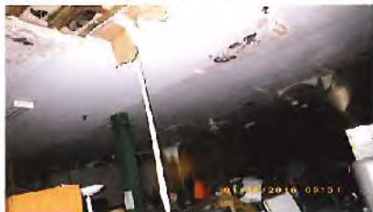
Ceilings full of mold and falling down in storage room
