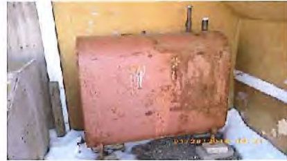
Oil Tank Older than 10 years
