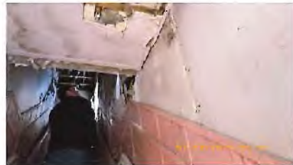
Walls destroyed due to moisture and vandals
