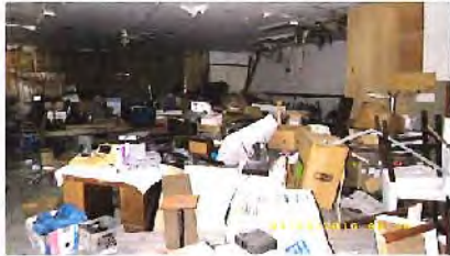
Large amount of combustible material and ceilings falling down in storage room
