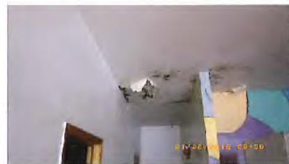
Mold on ceiling downstairs indicates leaking
