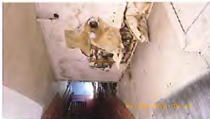
Stairway to upper floor ceiling has completely failed
