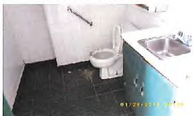
Downstairs Bathroom not functional water frozen in toilet
