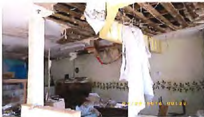
Ceiling is covered in mold and is falling down
